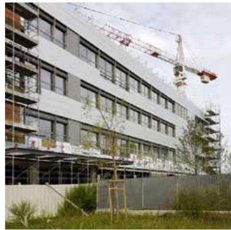
Siemens headquarters International competition, winner (green building award 2010) Client: Siemens S.p.A. Real Estate Milan 2007 / ongoing Project competition, preliminary and definitive design Project area: 180.000 m 2 ; built surface: 80.000 m 2
